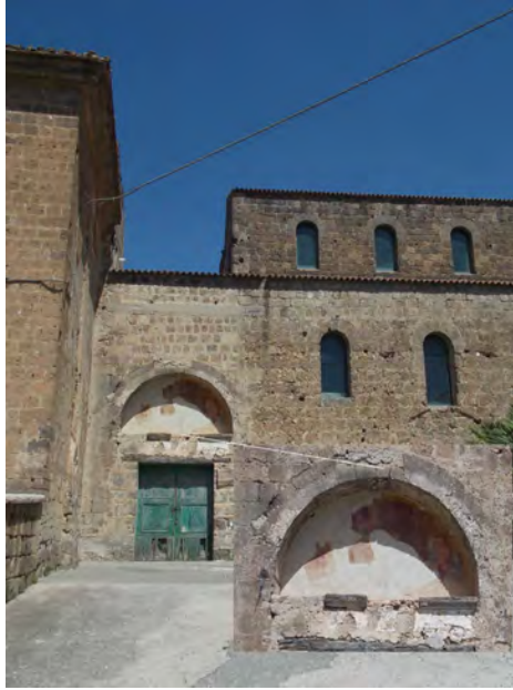
Fig. 4: Lateral access to S. Pietro ad Montes, which leads into porch. Zoom on the frescoed lunette.
